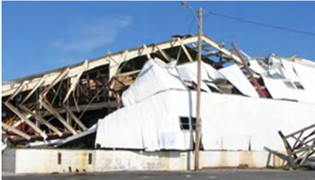
Fig 5.2.74: Warehouse disaster due to wind
