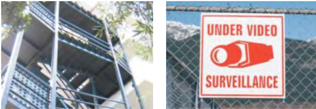
Fig 5.2.79: External emergency staircase & Peripheral fence with sliding gate
