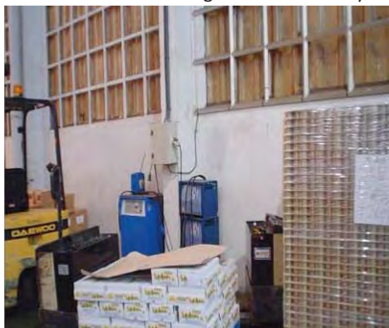
Fig 5.2.54: Material stored next to a battery charger
