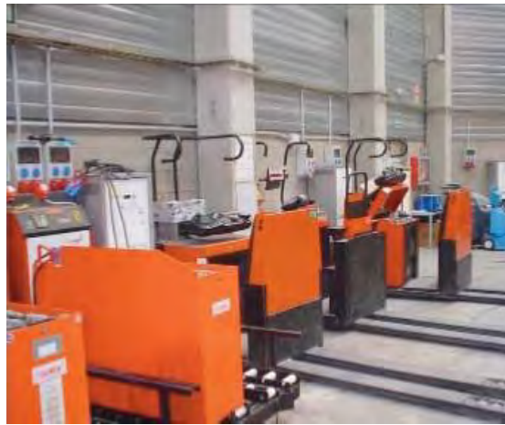
Fig 5.2.55: obstacle-free battery - charging area
