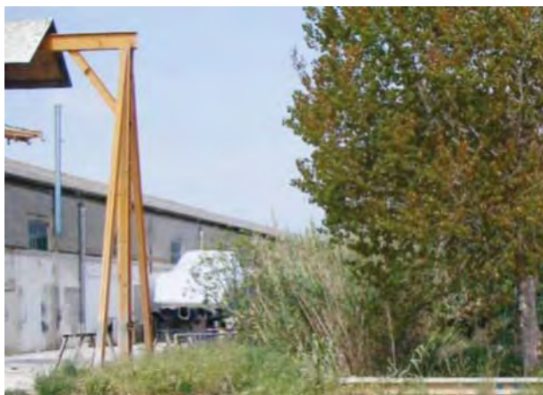
Fig 5.2.68: Undergrowth outside the warehouse increases risk of fire
