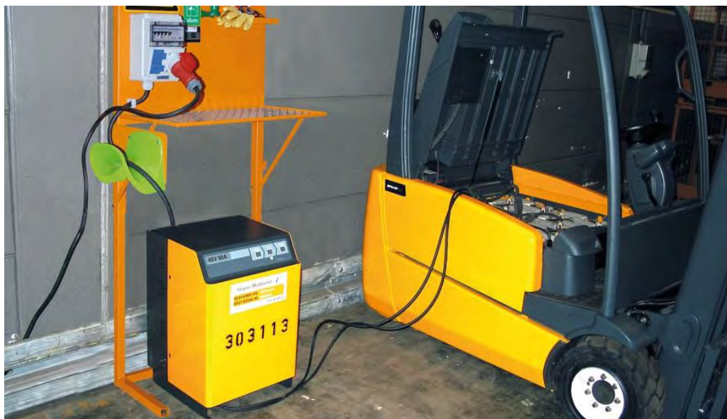
Fig 5.2.53: Forklift in direct contact while charging battery
