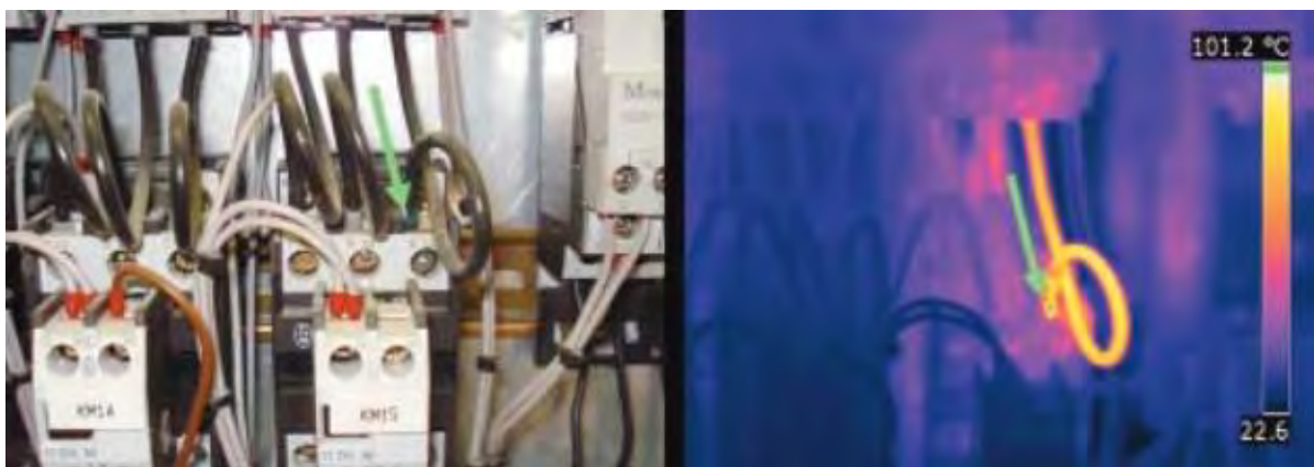
Fig 5.2.51: Thermal Imaging Analysis of a Main Switchboard. Real image on the left, thermal image on the right.
